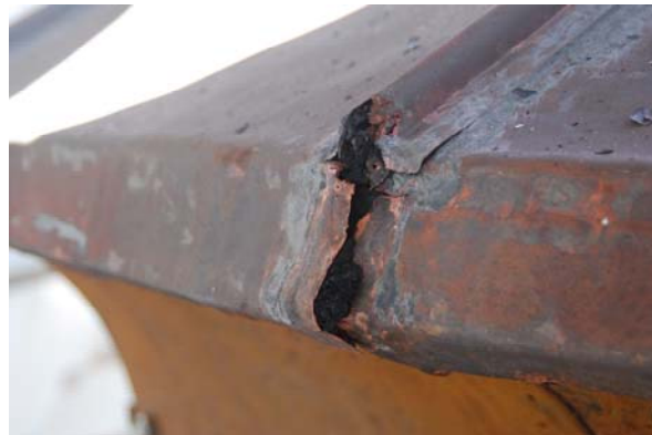
typical lighthouse roof damage (Nik Epanchin)
