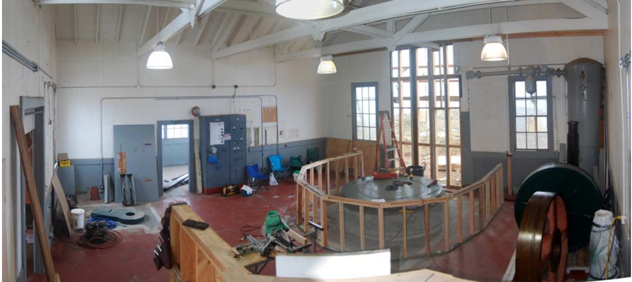
lens and drive foundations, west wall repairs and pony wall installations (Nik Epanchin)
